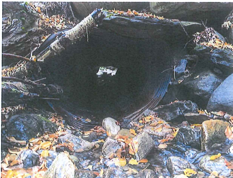
Photo 2 (25) Inlet Elevation Significant Culvert Damage/Debris Build-Up
