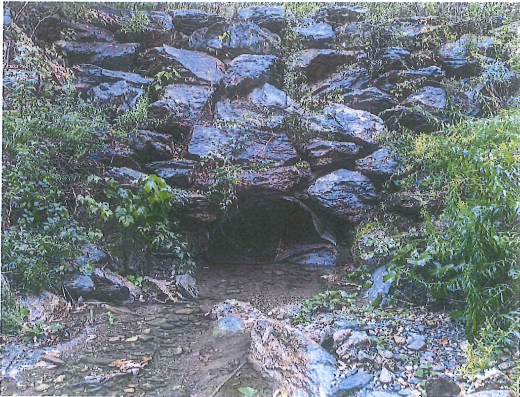
Figure 3: Culvert 25 - View of Crushed CMP Outlet (Handy Hill Road 0.26 Miles North of The Intersection with Bert White Road)
