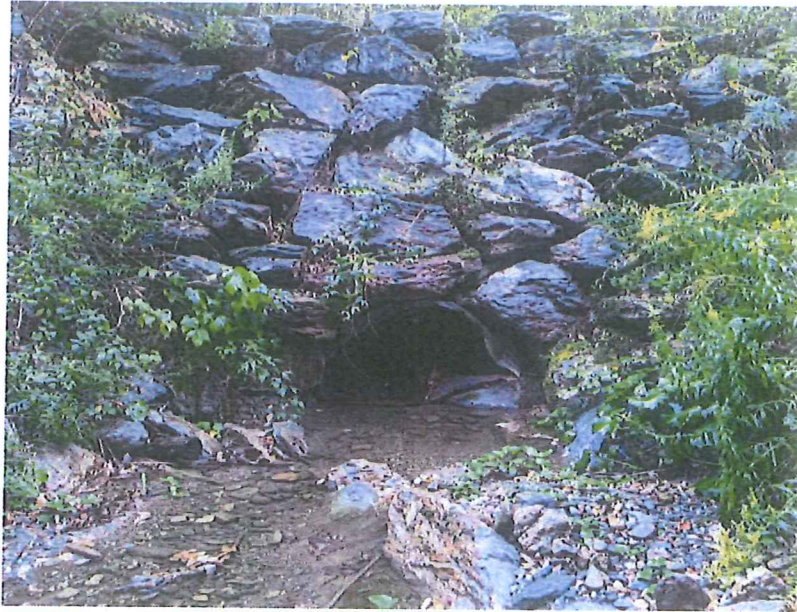
Photo 3 (25) Outlet Elevation Severe Culvert Failure (1/2)
