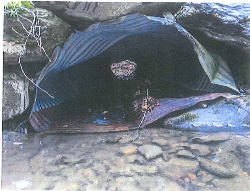
Photo 4 (25) Outlet Elevation Severe Culvert Failure (2/2)
